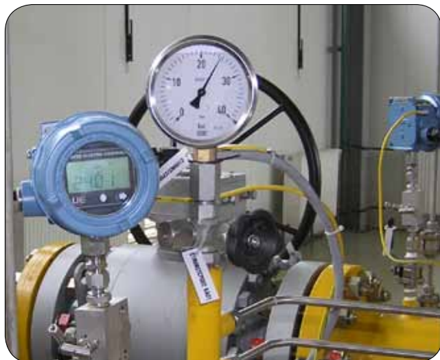
Pump Emergency Shutdown
