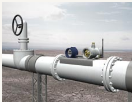
Landfill Gas Flow Control
