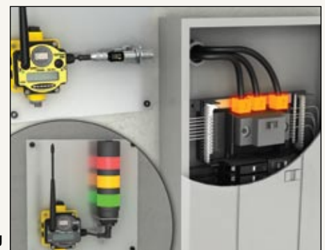
High-Temperature Alarm Conditioning
